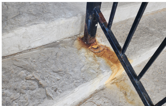
Rust staining, typical at steel posts
