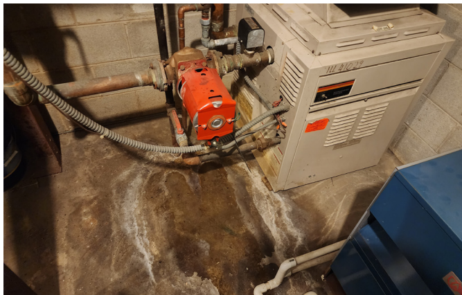
Boiler in basement
