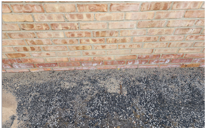
Water saturated brick along grade
