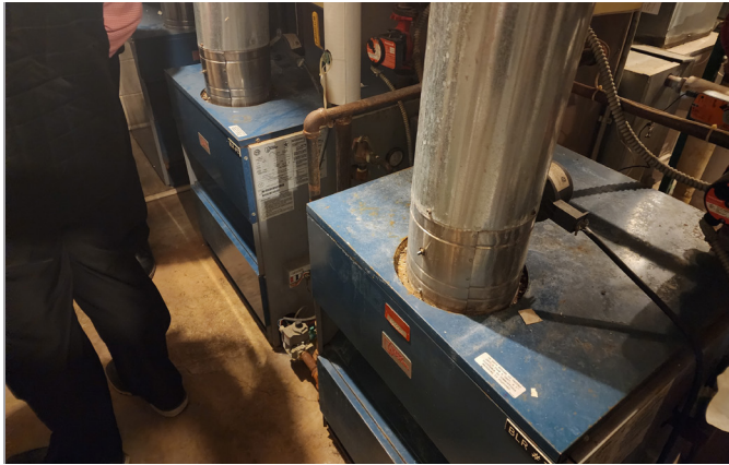
Boilers in basement
