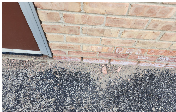
Spalled brick, loose mortar
