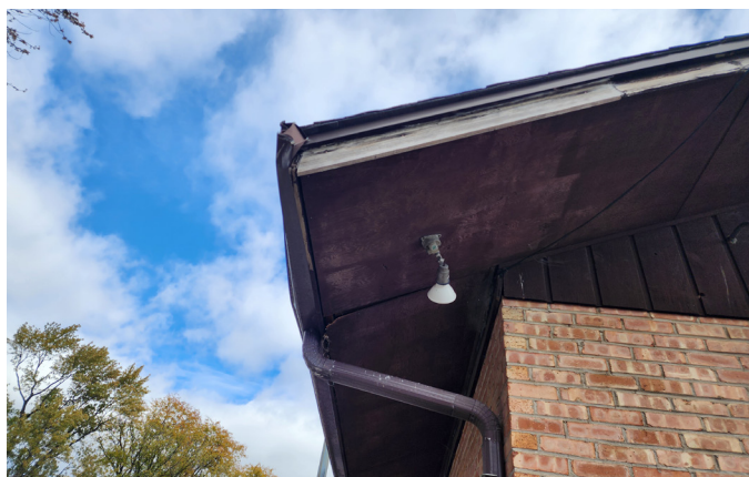
Damaged gutter, rotted fascia boards and open soffit
