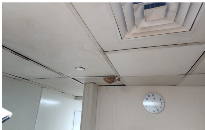
Water leak in kitchen ceiling
