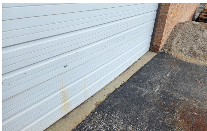
Bottom panel of overhead door damaged
