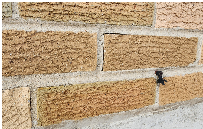
Loose and cracked mortar
