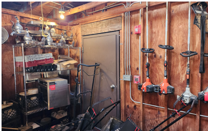
Exterior door and frame w/ daylight visible at perimeter of frame
