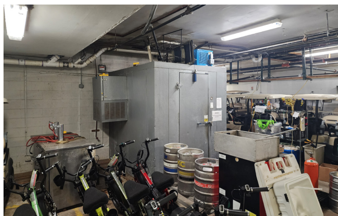
Beverage cooler in basement
