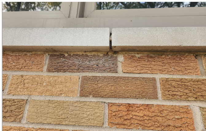
Mortar missing at sill; mortar loose at brick joints
