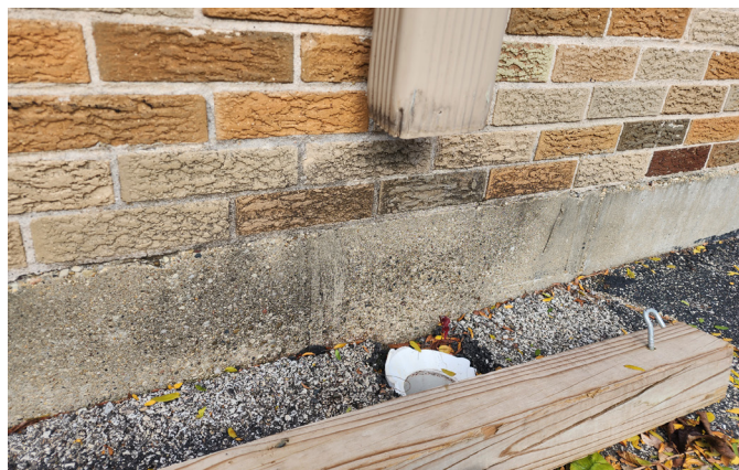
Connection to storm missing
