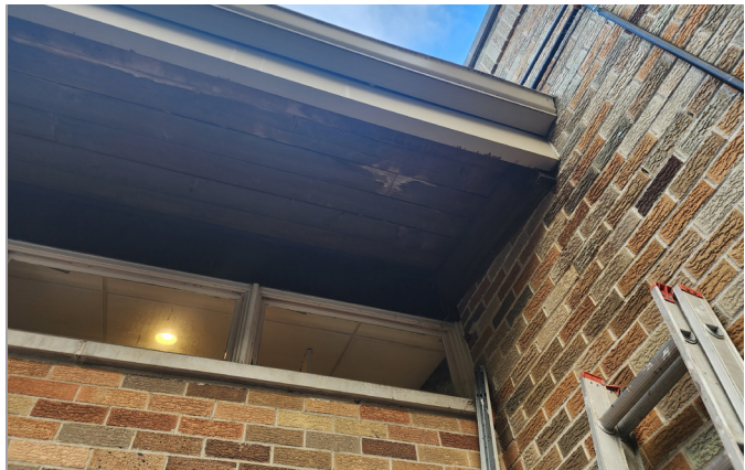
Water damaged soffit boards
