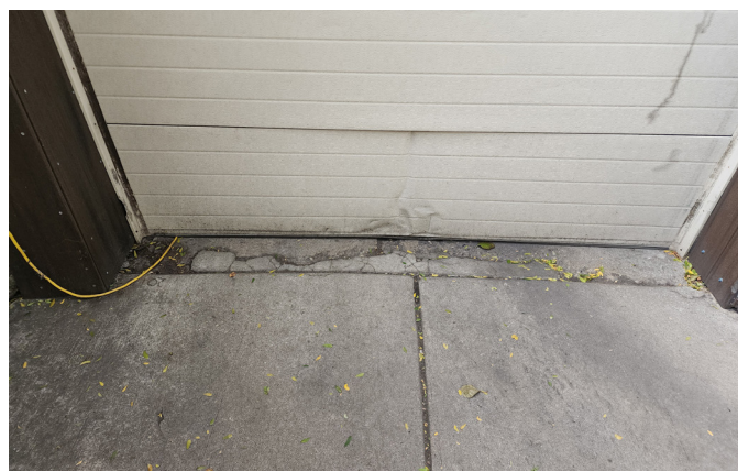
Damaged bottom panel at overhead door
