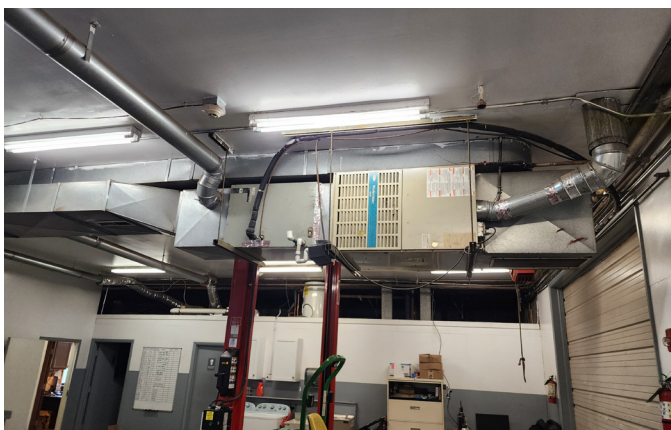
HVAC equipment serving all spaces less equipment bay
