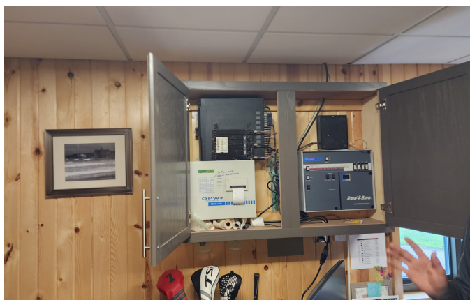
IT / Electric equipment housed in cabinet in office space
