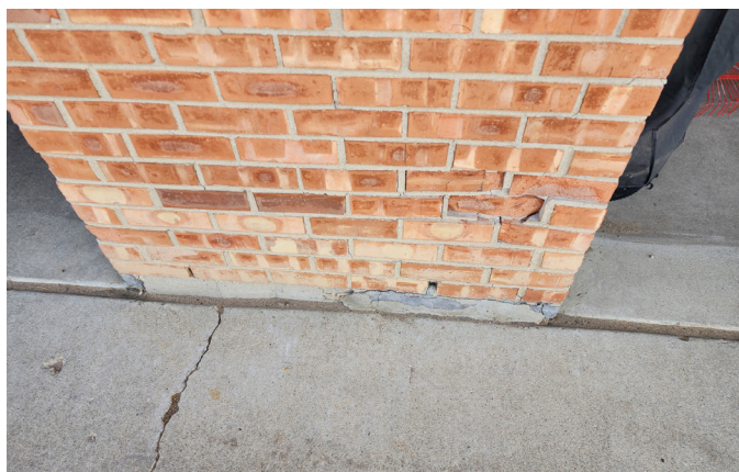
Spalled brick, cracked mortar, and damaged concrete
