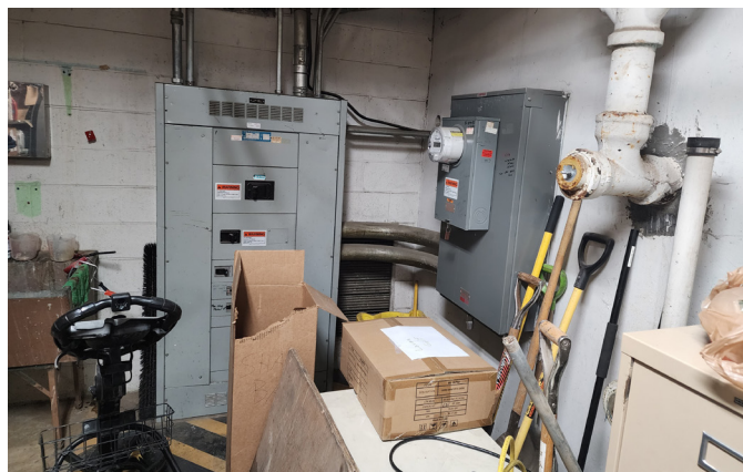
Electrical service entry
