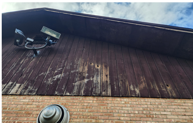
Weathered siding, soffit, & fascia
