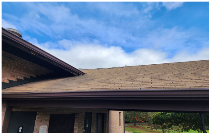
Missing shingles towards ridge, wear & staining observed where high roof dumps onto low roof
