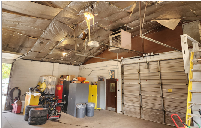
Equipment bay east
