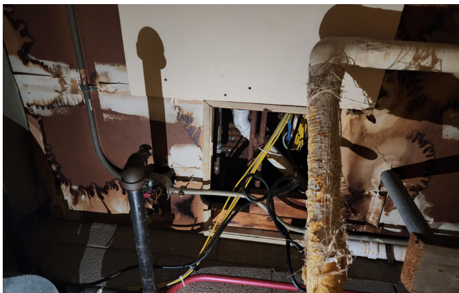
Exposed wiring, missing access cover; observable joists and deck showing signs of corrosion
