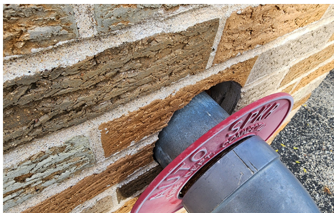
Mechanical penetrations not sealed
