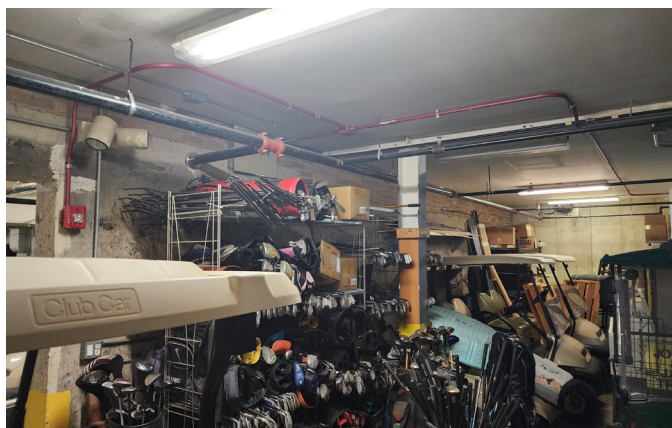
Bag storage in basement
