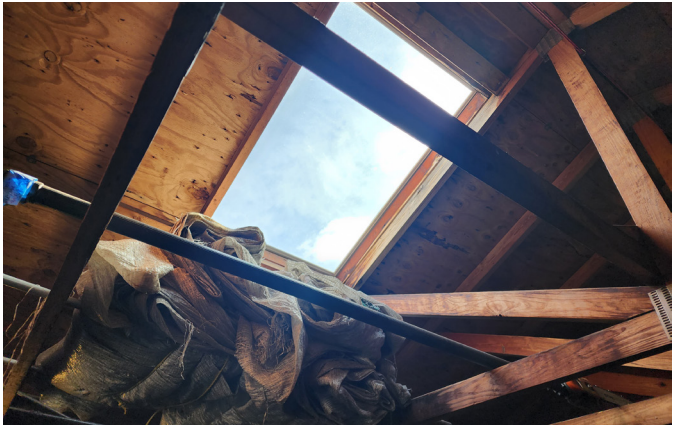
Water damaged truss
