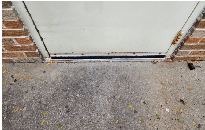
Rusted frame, hardware and door bottom
