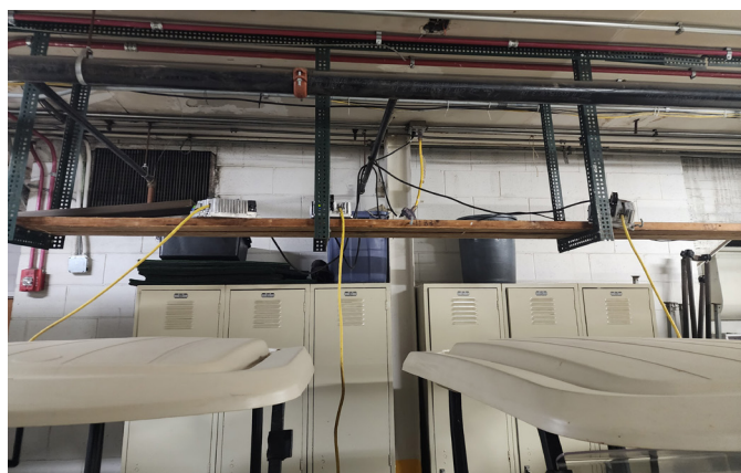
Cart charging equipment and rack
