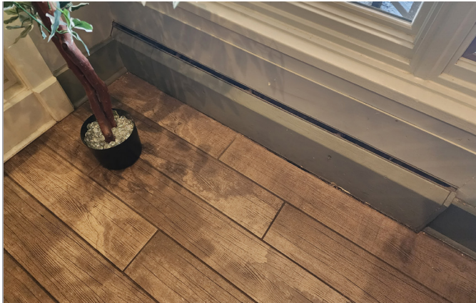
Baseboard radiant heat
