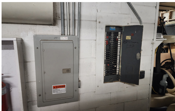
Electrical panels in basement
